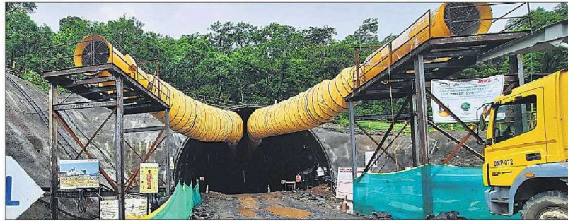
The NHSRCL is carrying out excavation work for the construction of the underground bullet train station.
